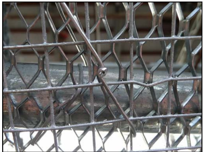
First of Two Layers: 1/2" 19 gauge welded wire mesh is placed and tied over the metal lath.
