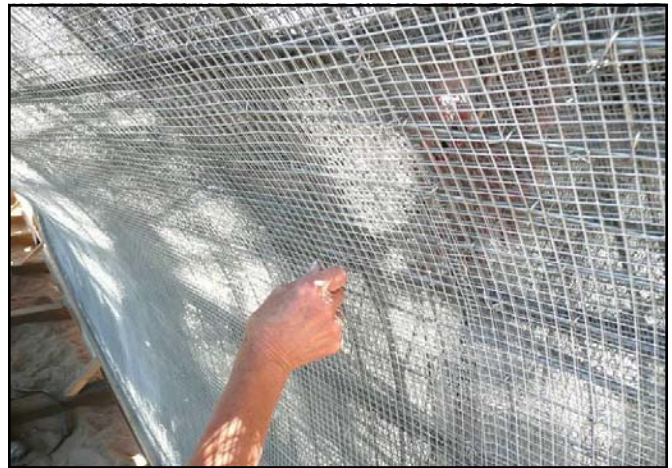
Final Step: The armature gets a wire twist at each 2.5" intersect formed by the 8 gauge wires
