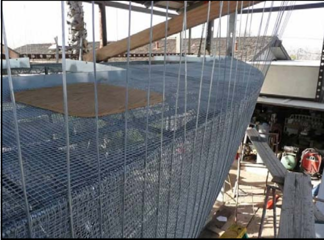
Wire Stringers: After the second layer of 1/2" w. w. mesh, the 8 gauge stringers are attached.
