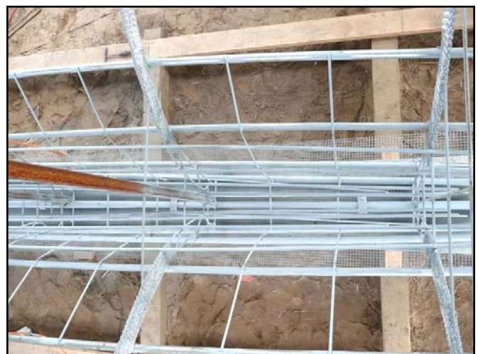
Keel: Steel rod & re-bar were welded in throughout then cold galvanized to resist corrosion.
