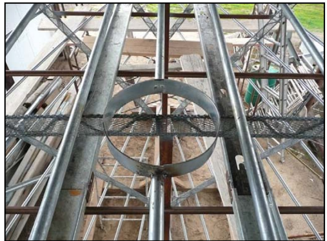
Mast Collar. The mainmast passes through this deck collar and steps onto the keel.
