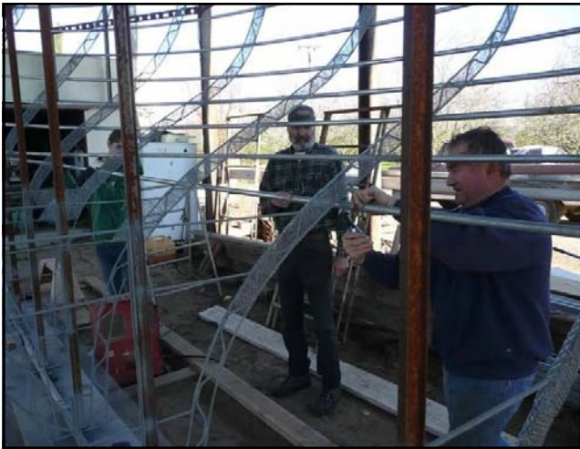
Longitudinals: 3/4" galvanized pipe were first wired on, then welded to the frames.
